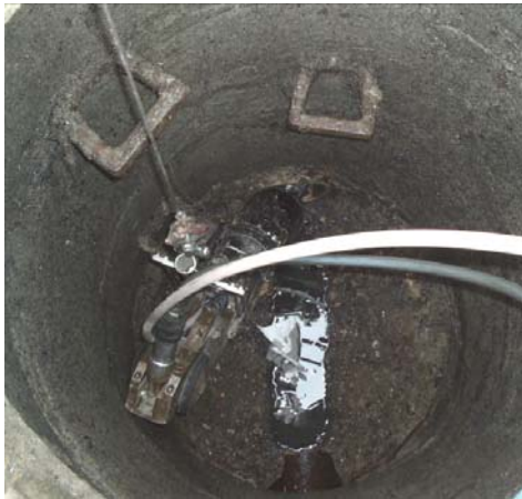
Fig. 9: Attempt to use a satellite camera through a shaft in a DN 200 pipeline
